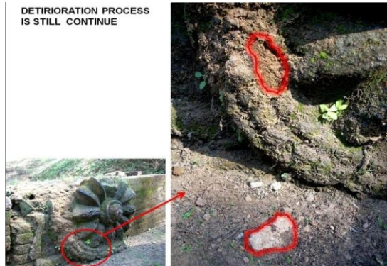
Figure15. On site example of stucco flaking, Nalanda archaeological site, Nalanda, Bihar (Right)
