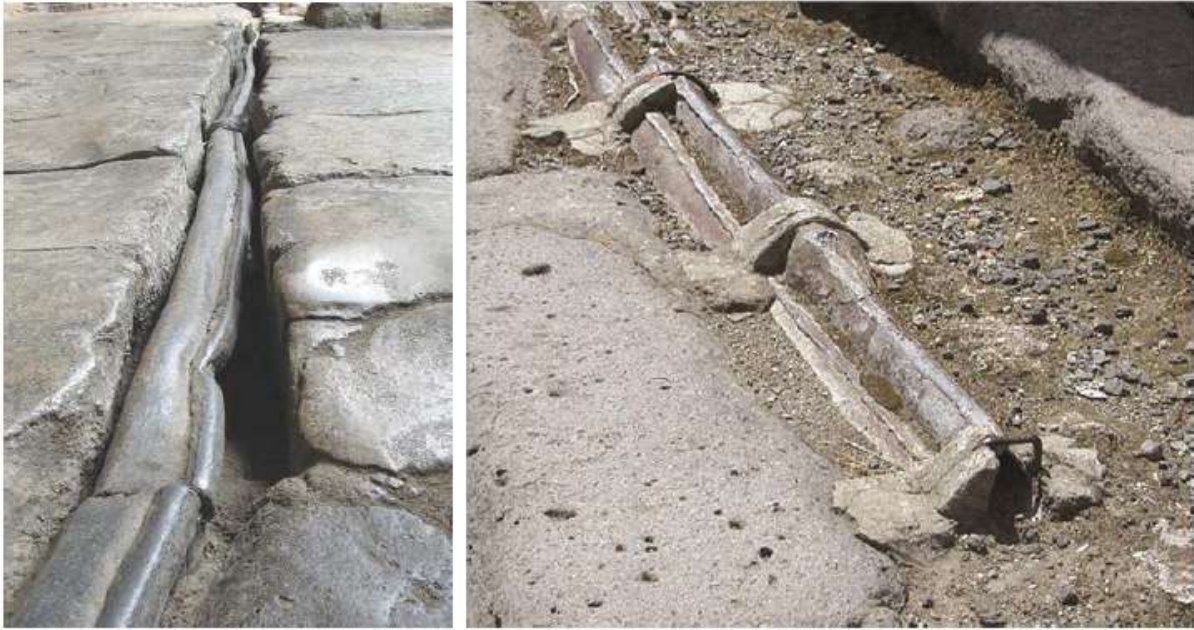
Figure14b. On the upper part of the pipes are signs of the longitudinal welding, the result of the process for curving a metal plate rather than drawing.
