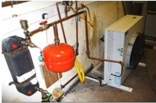
Fig3. Shows the connections of the heat exchanger, water pump, heat rejection fan and expansion valve.
