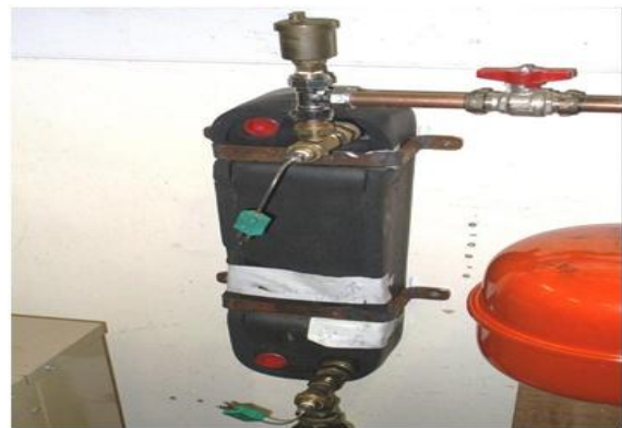
Fig2. Shows the heat exchanger
