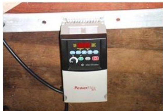
Fig5. Shows the power supply to heat injection fan
