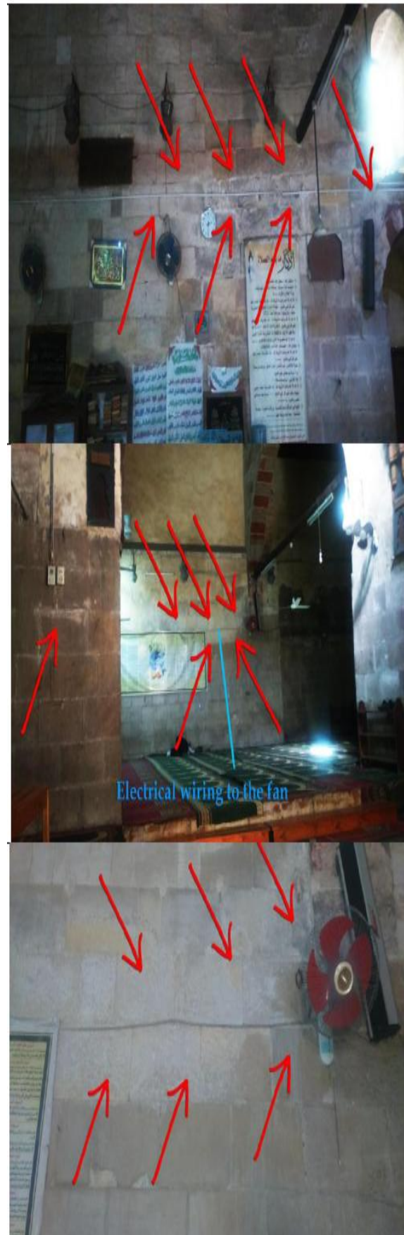
Figure9. Top, middle, and bottom (Zoom in) pictures, are showing "Efflorescence" forming around plastic conduits, and fans installed over lime stone walls of the prayer hall inside "Prince Timraz Ahmadi" mosque. Reference: [Researcher].
