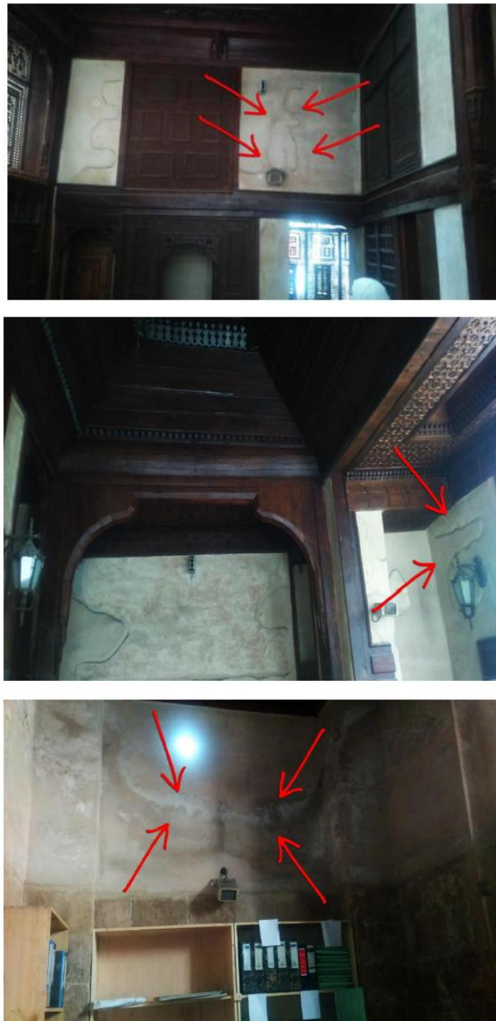
Figure12. Top, Middle, Bottom pictures are showing "Efflorescence" forming around sound speakers, and electrical lanterns inside the "Haramlek", and also around wiring extensions embedded inside the wall crevices of the surveillance control room at the ground floor of the house of "Sheikh Abu El-Anwar Al-Sadat". Reference: [Researcher]
