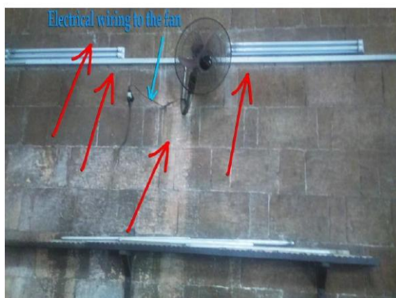
Figure7. Top and Bottom pictures are showing "Efflorescence" forming around plastic conduits, and fans installed over lime stone walls of the prayer hall inside prince "Zulfikar" mosque, Reference: [Researcher]
