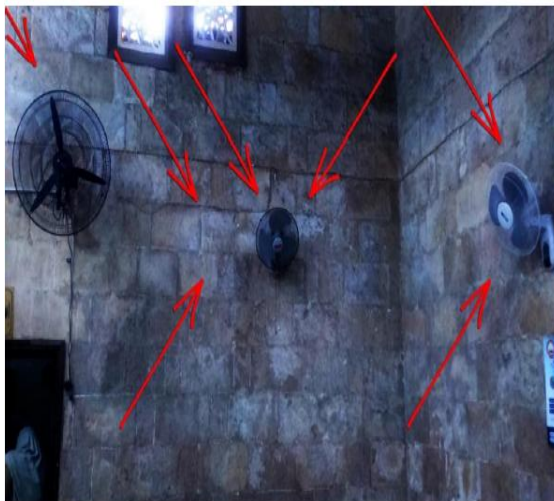
Figure19. Top and Bottom Pictures are showing the formation of "Efflorescence" around bare electrical wiring extended to fans over the walls of "Hassan Pasha Taher" Mosque prayer hall. Reference: [Researcher]
