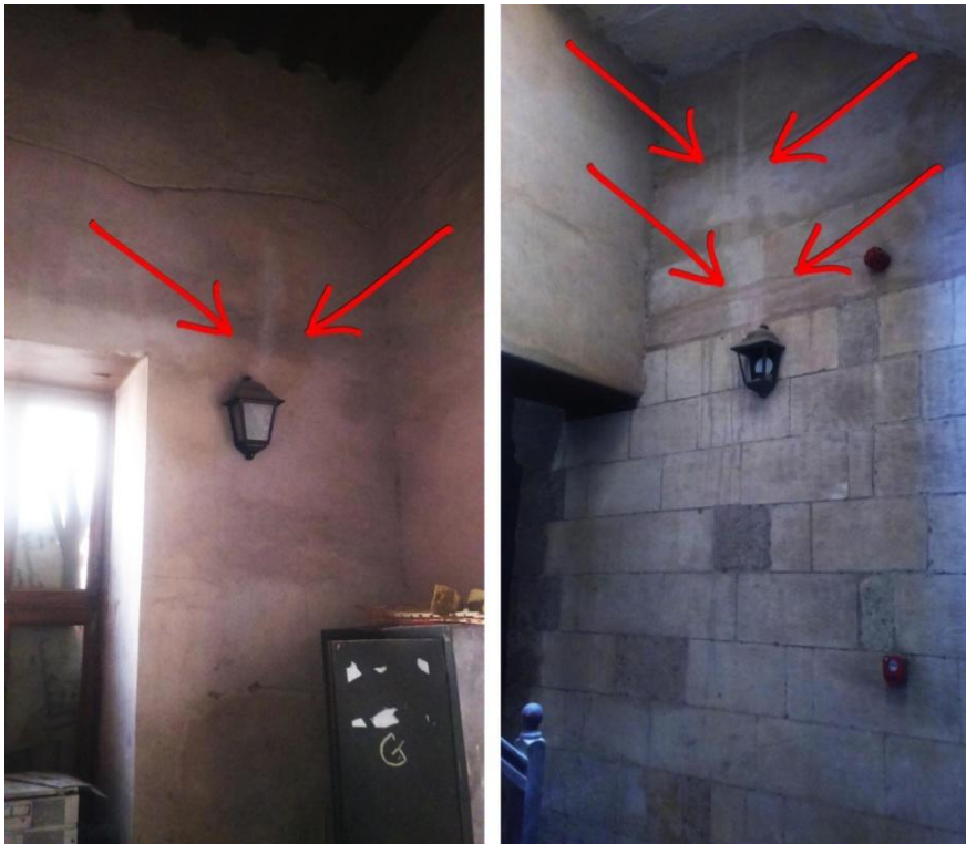
Figure13. Is also showing "Efflorescence" forming around installed electrical lanterns inside the "Sheikh Abu El-Anwar Al-Sadat" staircase. Reference: [Researcher]
