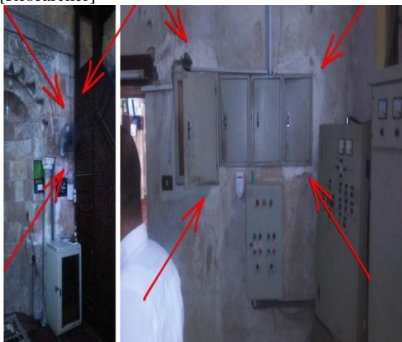
Figure20. Left and right pictures are showing the formation of "Efflorescence" around the fan installed at the "Mihrab", and around a series of electrical panels that are found in "Hassan Pasha Taher" Mosque electromechanical room. Reference: [Researcher]
