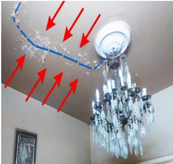
Figure 5. Shows "Efflorescence" accumulated under a painted ceiling of the saloon in the same apartment presented above. "Efflorescence" formed around electrical conduits that are embedded in the grouted crevices leading to the ceiling chandelier. Reference: [Researcher]
