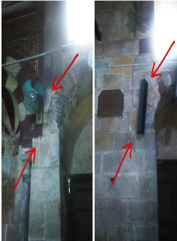
Figure15. Shows the formation of "Efflorescence" around sound speakers installed over the lime stone walls of the "Mustafa Fadil" Pasha mosque entrance lobby. Reference: [Researcher]
