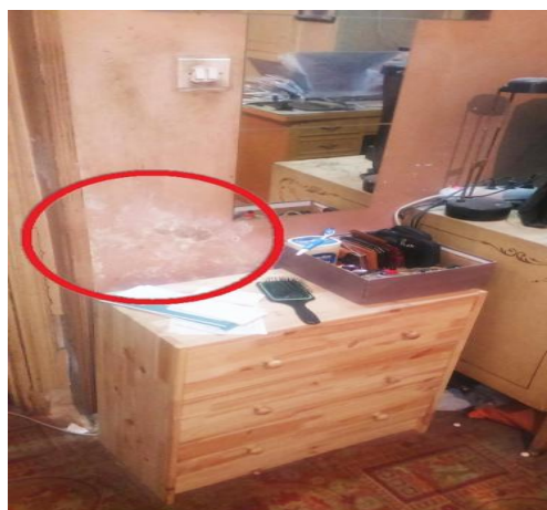
Figure2. Shows "Efflorescence" on the interior walls of a modern apartment in Egypt, Shows the effect almost reaching the top of the bathroom walls from
