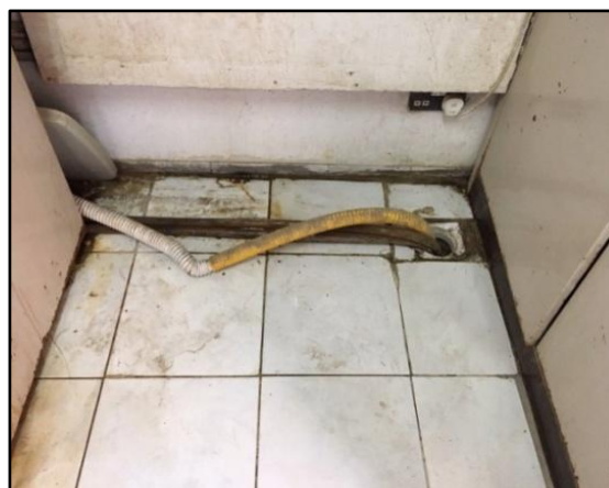
Figure 4. The damaged and blocked pipe from the sink goes to the drain.
