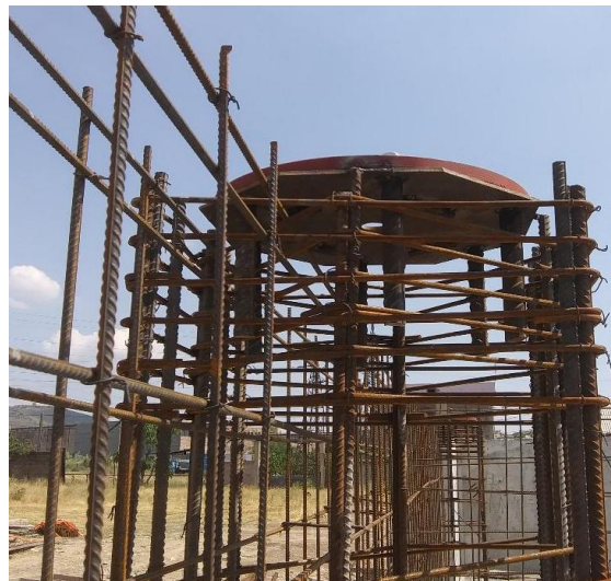
Figure9. View of the lower socket on top of the lower pedestal for location of SILRSB
