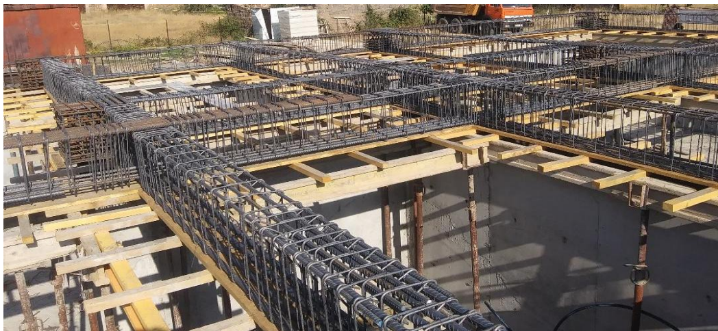
Figure13. Reinforcement frames of beams are installed and passing through the reinforcement frames of upper pedestals
