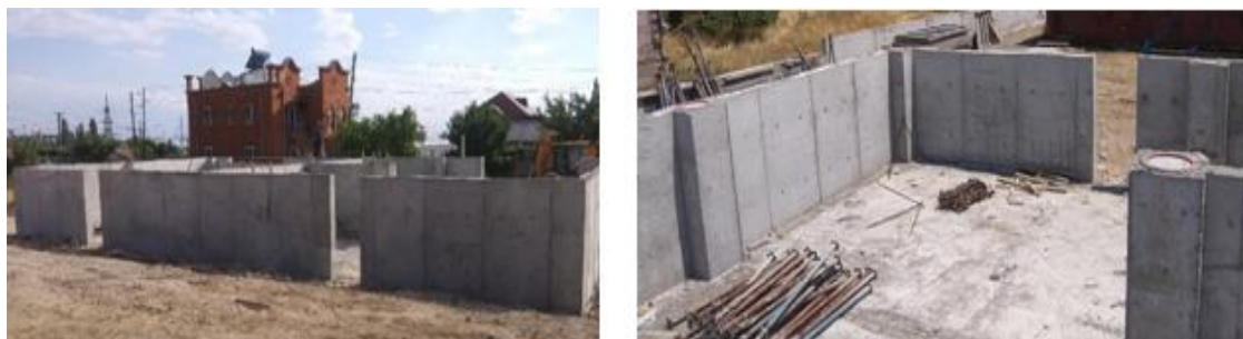
Figure10. Views of the concreted shear walls, lower pedestal and of SILRSBs' lower sockets on top of them
