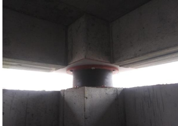
Figure 14. View of the SILRSB installed in the lower and upper sockets between the lower and upper pedestals at the corner of the building
