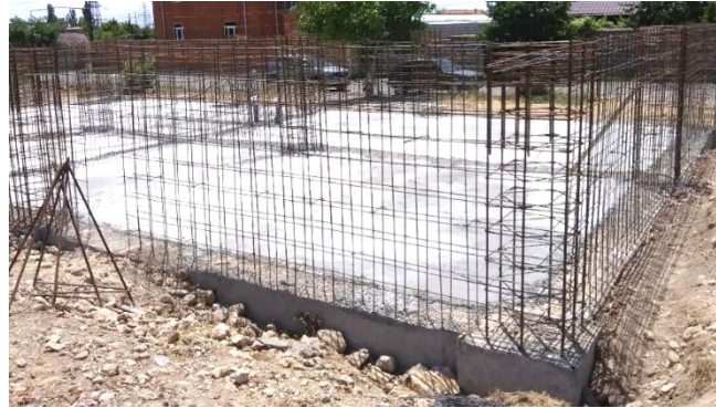
Figure8. View of the concreted foundation and the reinforcement frames of the lower pedestals and the shear walls
