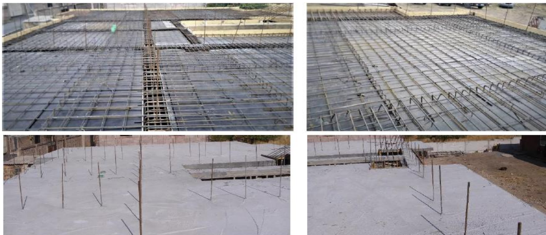
Figure 16. Fragments of the reinforcement of R/C slab and their views after casting the concrete
