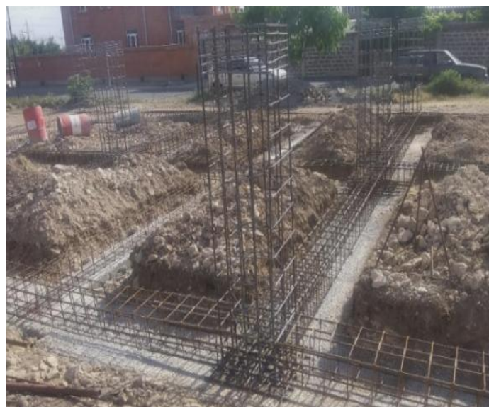
Figure7. Reinforcement frames of the lower pedestals and the continuous beams before installation of the shearwalls' reinforcement
