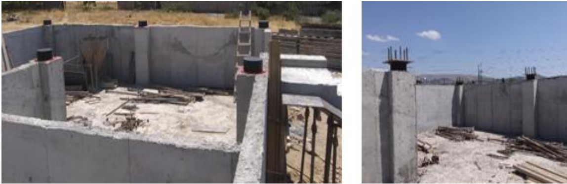
Figure11. SILRSBs are installed in lower sockets and then the upper sockets are placed
