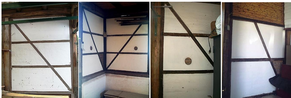
Figure16. Actual state of E.W's wattle and daub walls
