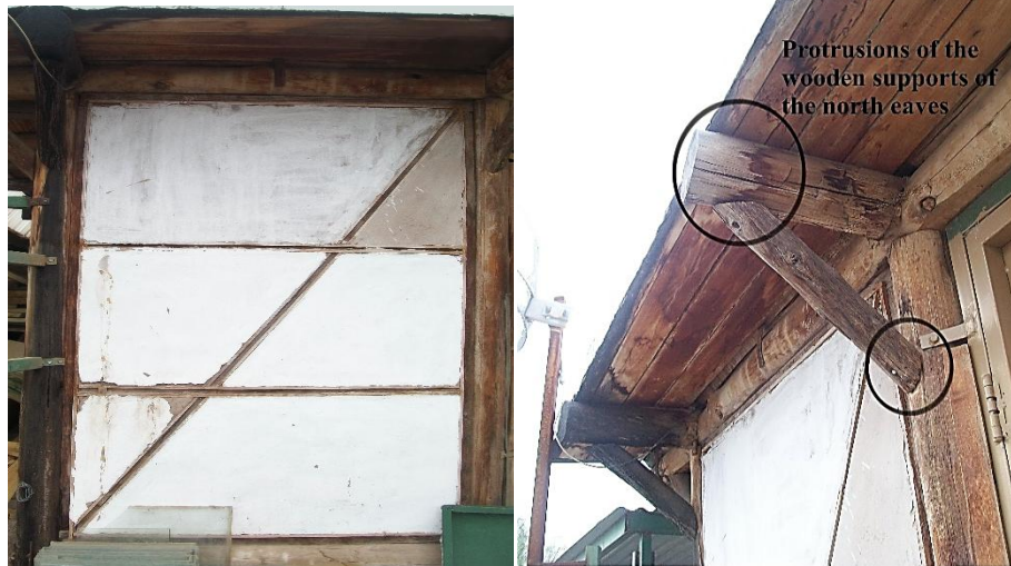
Figure 12. Pathologies in front north-facing wattle and daub panels of the E.W.
