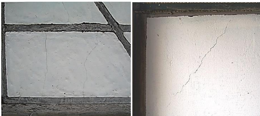
Figure15. Microcracks on wattle and daub walls.
