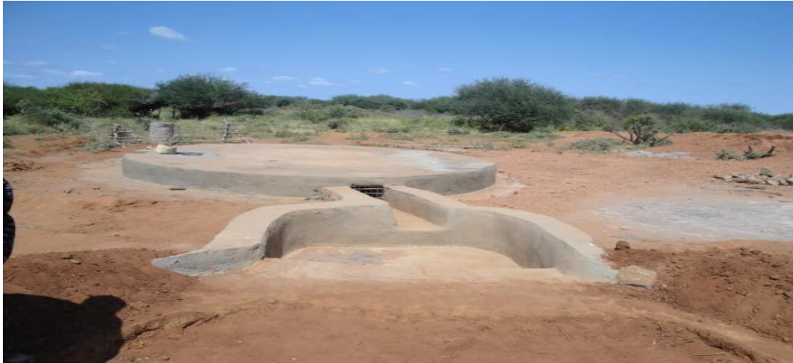
Figure3. Underground construction of the water cistern by some of the community at Yabello
